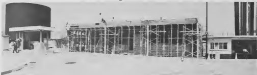
New headquarters for Industrial Services under construction, with part of present facilities at right.
